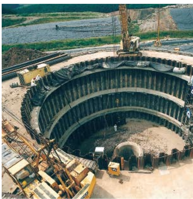
Regeneration drain at Asslar landfill
