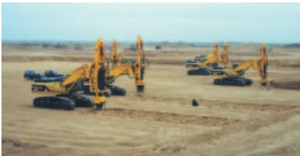
Six BSP Rapid Impact Compactor working in Kazakhstan on oil and gas plant
