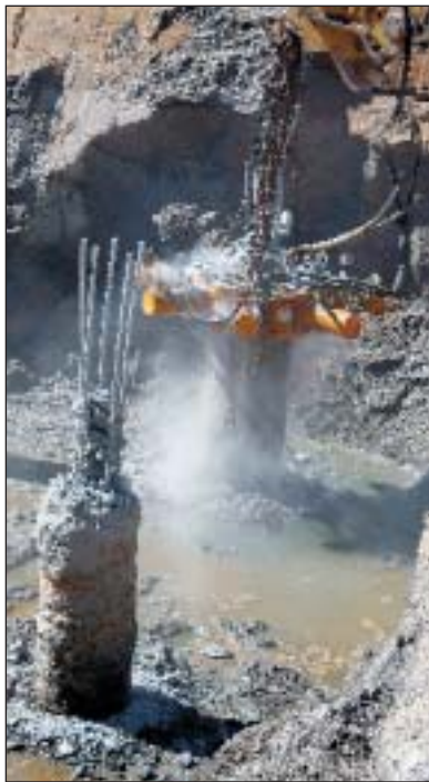
A Taets hydraulic pile breaker was used to trim piles to size and expose reinforcing
